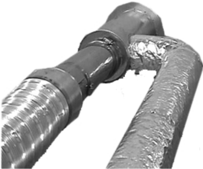
Figure 4 - Inside View of Vent Terminal
