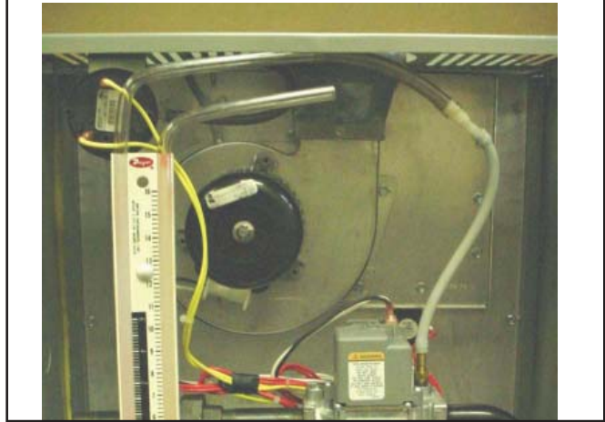
FIGURE 14 - MANOMETER MEASURING MANIFOLD GAS PRESSURE
