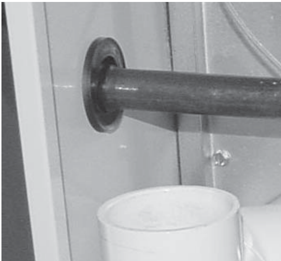
Figure 23 - Furnace Gas Pipe Connections (Note Rubber Grommet)
