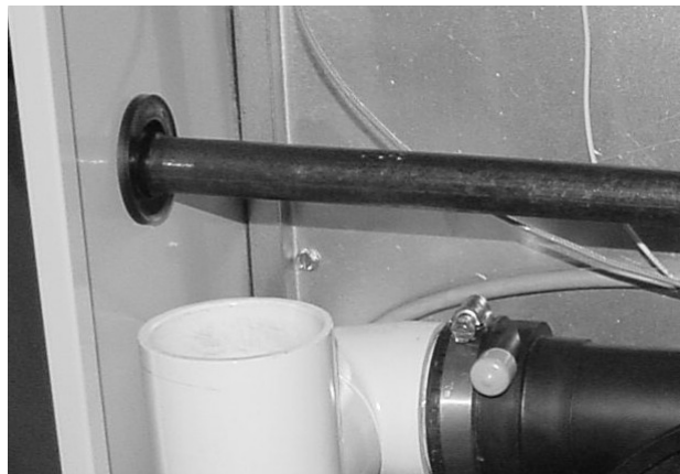
FIGURE 28 - FURNACE GAS PIPE CONNECTIONS (NOTE RUBBER GROMMET)
