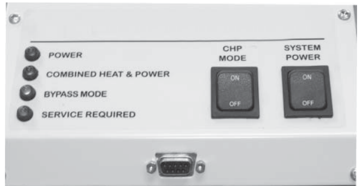
Figure 14-3 120 VAC System Power Switch
