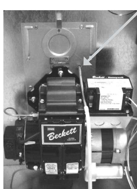
Over-fire draft access port.
