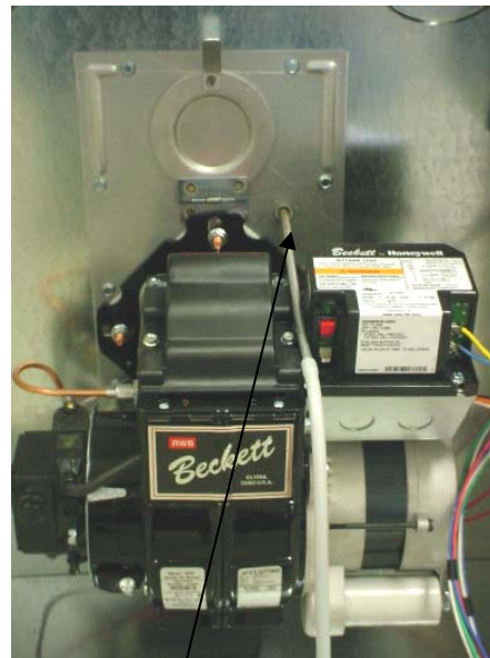
Over-fire draft access port.
