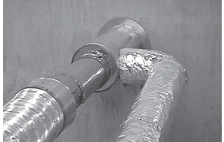
Figure 4 - Inside View of Vent Terminal
