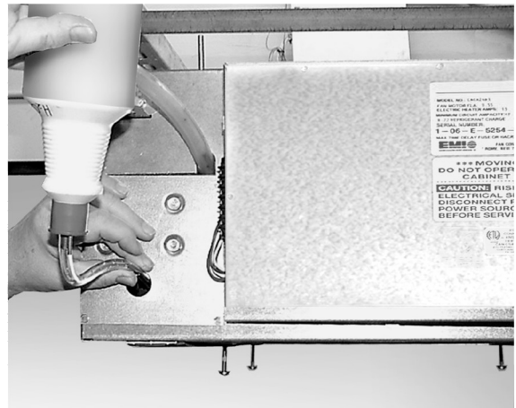
Figure 34 - Check Condensate Pump Operation
