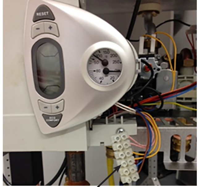
Low Voltage Terminal Strip Removed
