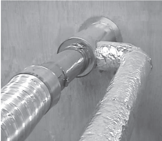
Figure 4 - Inside View of Vent Terminal
