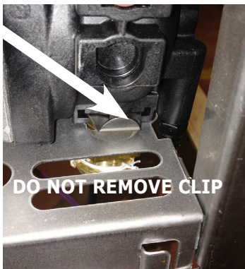
RIGHT SIDE CLIP - INSIDE BOILER JACKET
