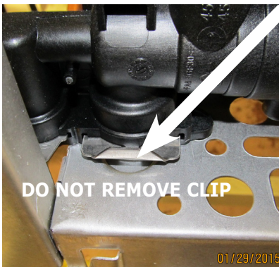
LEFT SIDE CLIP - INSIDE BOILER JACKET
