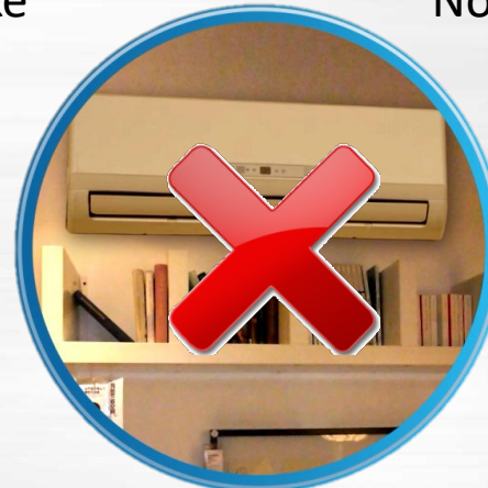
To close to ceiling preventing proper airflow
