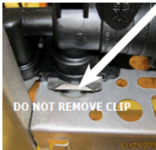
LEFT SIDE CLIP - INSIDE BOILER JACKET
