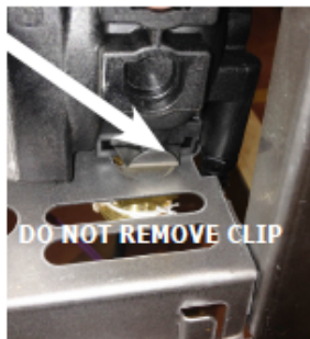
RIGHT SIDE CLIP - INSIDE BOILER JACKET
